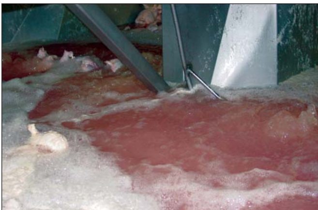
Chiller before adding Spectrum™
